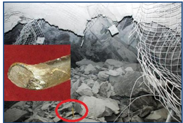
Ground support failure associated with seismic event
